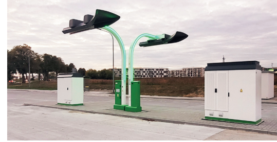
Flea 4 EVSE implemented in a charging station
